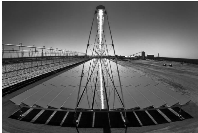
Figure 1. A typical LFR system (AREVA Solar's Compact Linear Fresnel Reflector)
